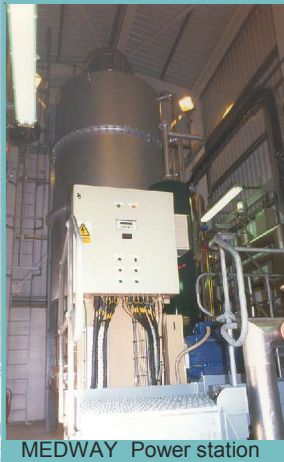
MEDWAY Power station (U.K.)
